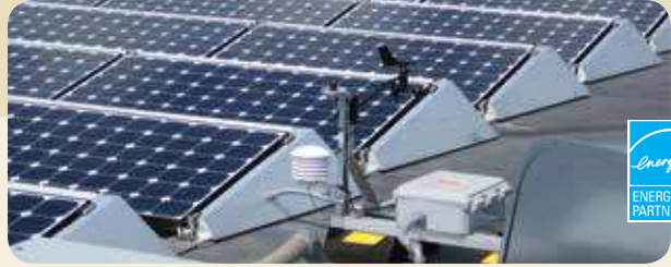
Photovoltaic roof panels, New London, CT branch
